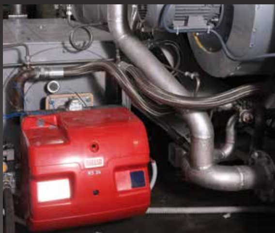
Gas Heating System
